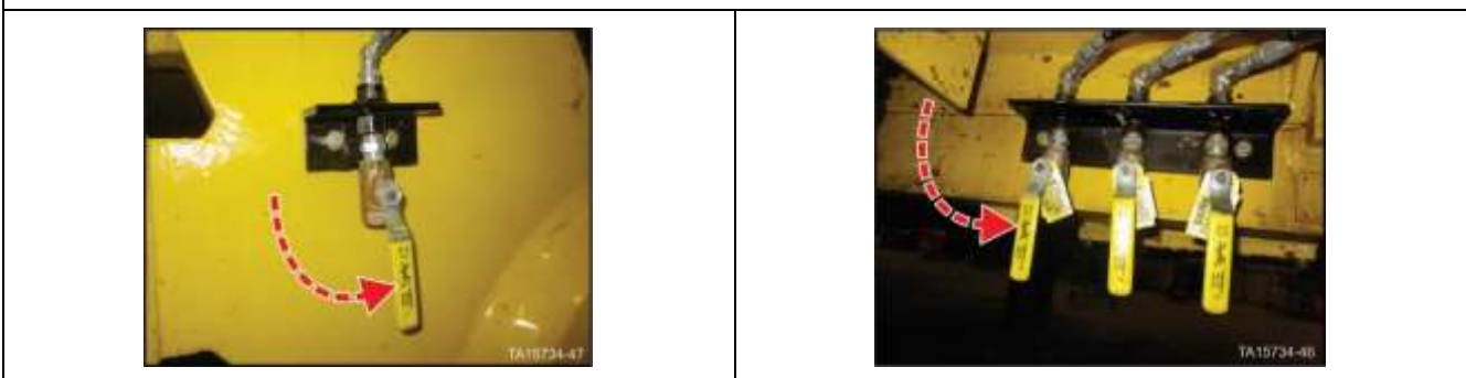
Open air reservoir bleed valves
