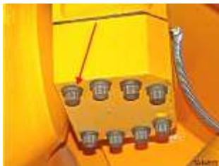
Arrow indicates location to be cleaned
