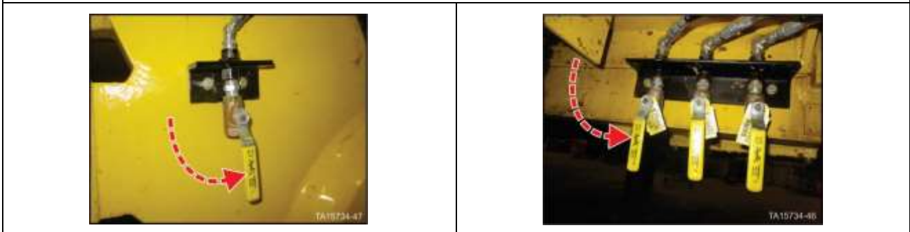
Open air reservoir bleed valves
